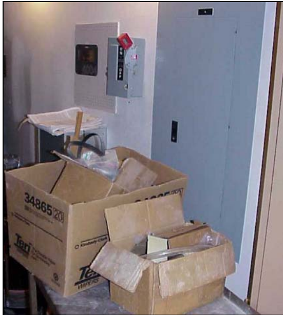
Improper Storage in front of Electrical Panel
