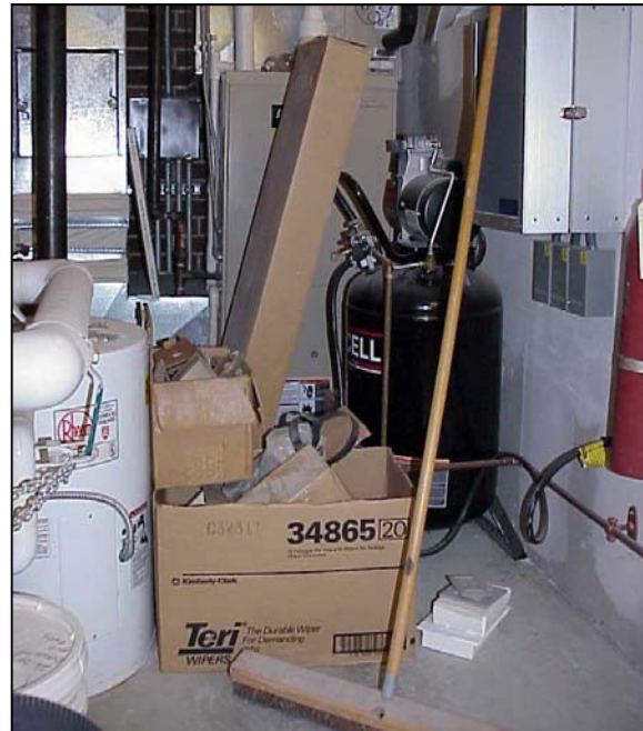
Improper Mechanical Room Storage
